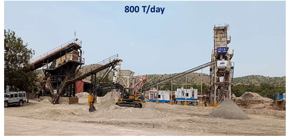
Steel slag sand manufacturing unit
