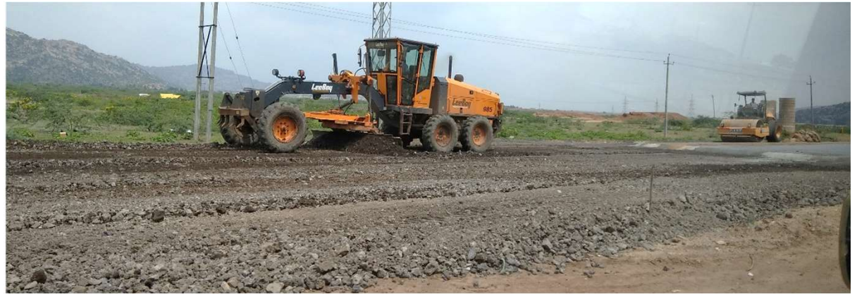
NH-67: Hosapete to Ballari: Total Length 95 KM Concrete road made up of slag aggregates (Fine and Coarse)
