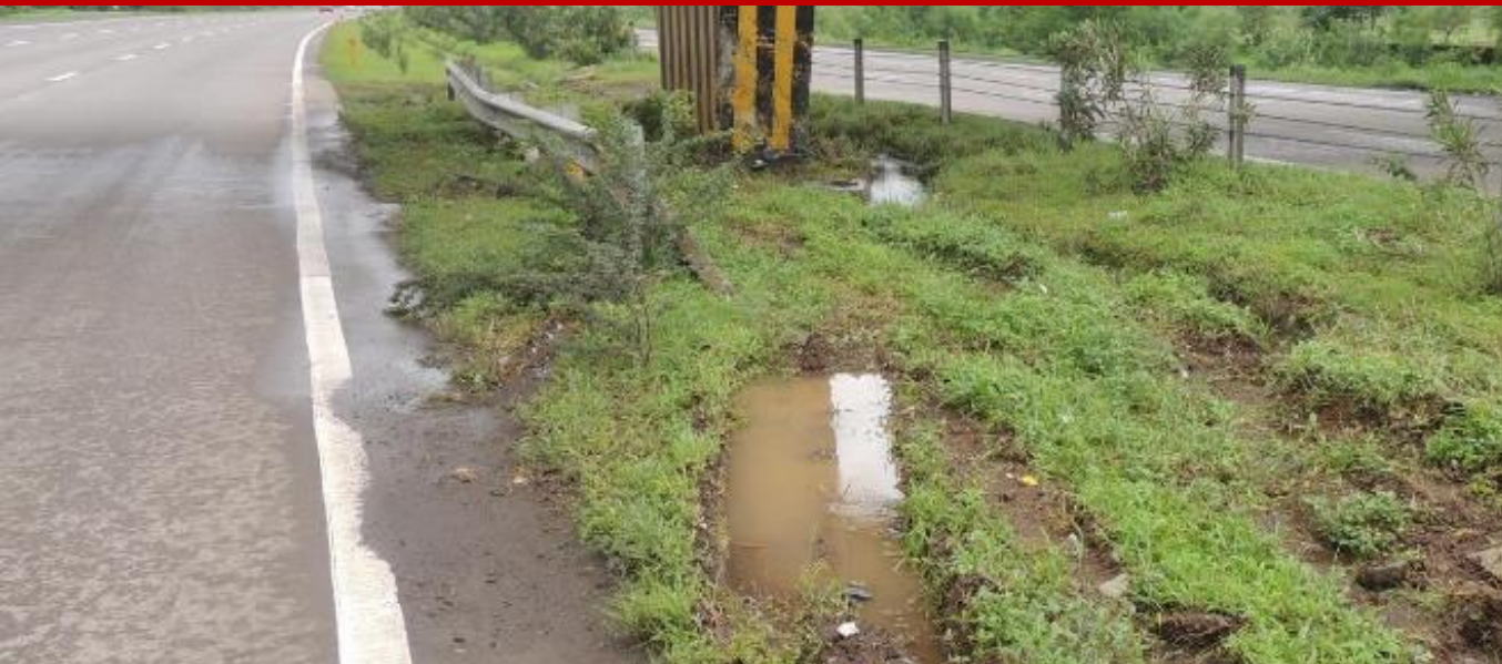
Guardrail run-out length too short
