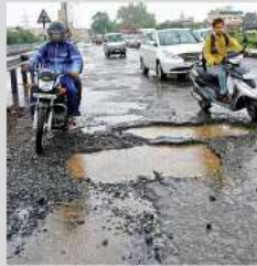
Poor Quality Road Infra
