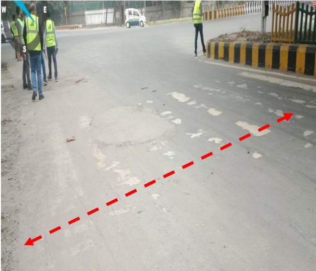
No proper signs and marking indicating crossing
