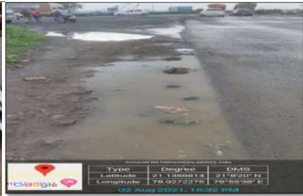
Damaged shoulder at Ch 18+050 LHS
