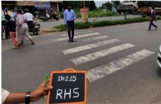
Cat-eyes not fixed near pedestrian crossing & median opening at ch 19+215 RHS
