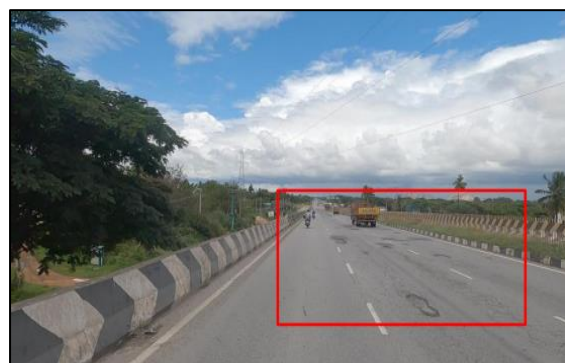
During Audit it is observed that pot holes are there on the carriageway
