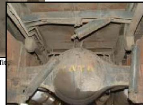
Shock absorber not fitted
