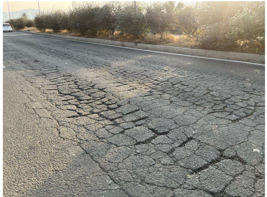
Typical pavement condition where White topping should be avoided
