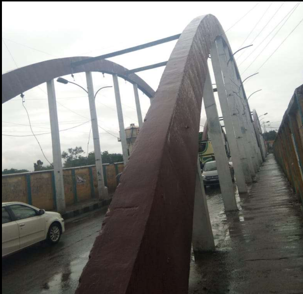
Cracks and delamination of cover concrete on Arch member
