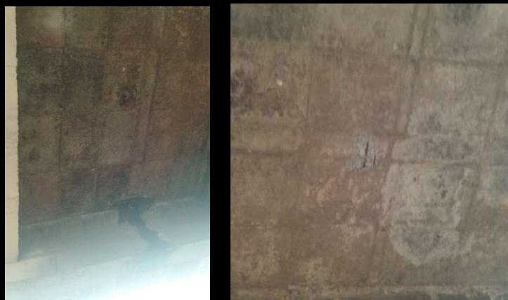
Spalling of concrete in the deck slab
