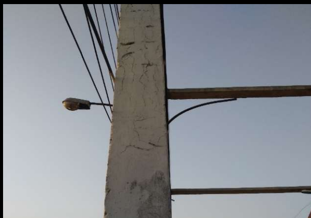
Cracks on hangers.
