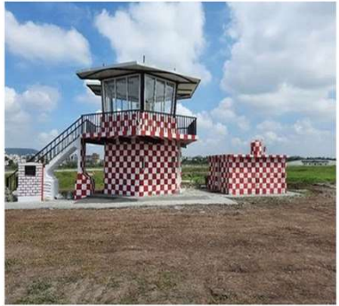
MiCoB delivers 3D Concrete Printed Runway Controller Hut for the Pune Air Force Station
