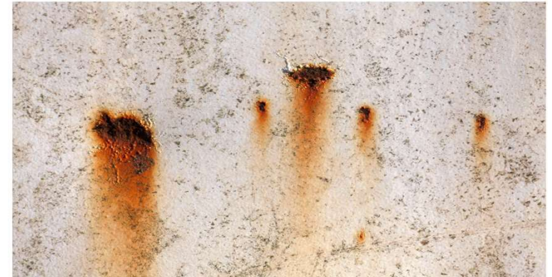
Corrosion Stains in Concrete
