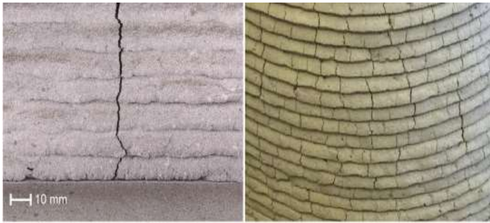
Shrinkage cracks in 3D printed elements (Moelich et al. 2020)
