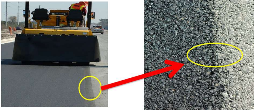
Tight Longitudinal Joints
