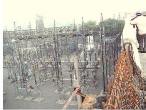
MAJOR ELECTRIC SUB STATION
