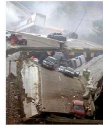
I-35 Bridge Collapse in Minnesota, US (2007)
