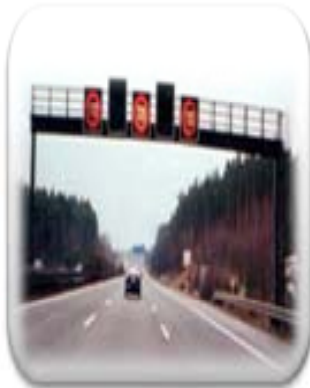
Speed Control Signs
