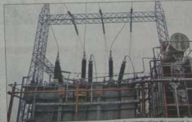
ANOTHER HITCH: UP Transco, which is responsible for constructing the project, is unable to transport heavy machinery and equipment to the site
